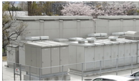
NaS batteries introduced by Pioneer Micro Technology
