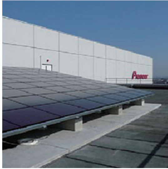
Photovoltaic system at Pioneer's Kawagoe Plant
