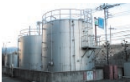
Oil barrier around crude oil tanks (Pioneer Micro Technology Corporation)
